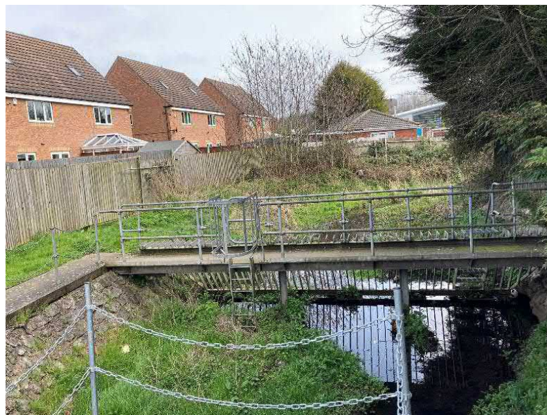
Figure 17: Site Visit Photograph - Double EA trash screen at the inlet to the culvert beneath Brook Road
